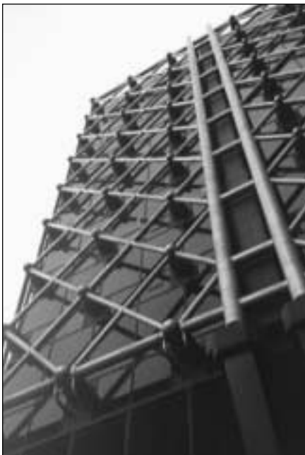
Structural tubes, filled with water, used as an external fire prevention system.
