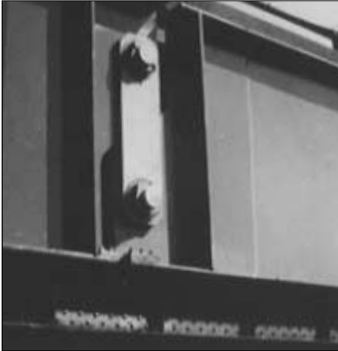
The Minnesota Department of Transportation replaced conventional low alloy steel with stainless steel hinge pins and hangers on the Blatnik Bridge in Duluth, Minnesota.
