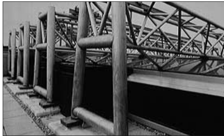
Stainless steel trusses (20 meters) for bracing and end frames for skylight supports.
