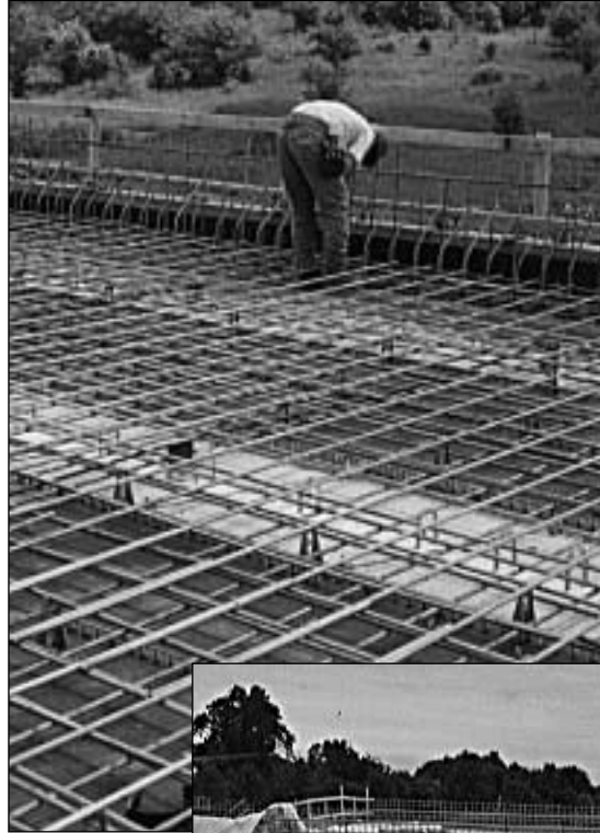
Stainless steel rebar being installed in a bridge on highway 407 in Ontario, Canada
