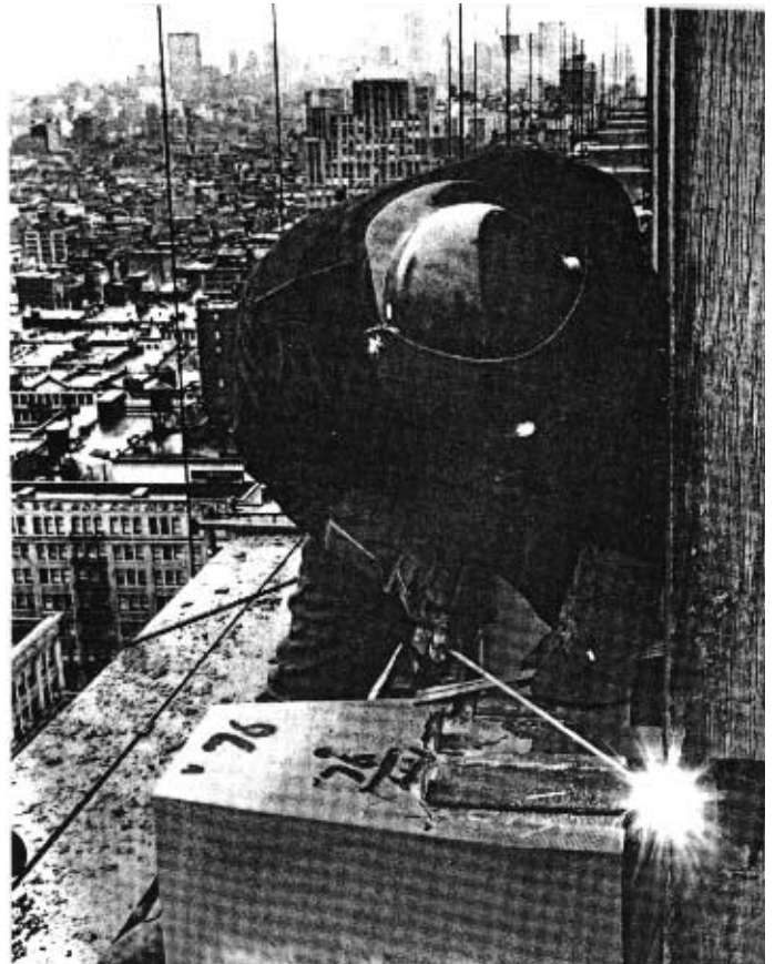
Two intermediate anchors are a split-tail design made from 1/4" thick stainless steel plate, 3" wide. Small-diameter stainless steel wire anchors serve to hold the limestone mullion until the anchors are welded to the structural steel.
